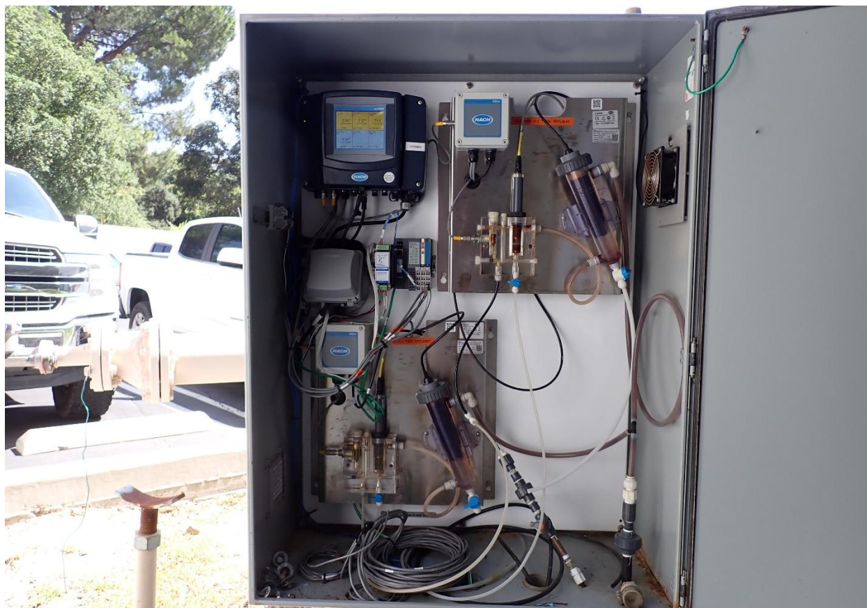
Figure 5.3 Well 10 Water Quality Sampling Cabinet
