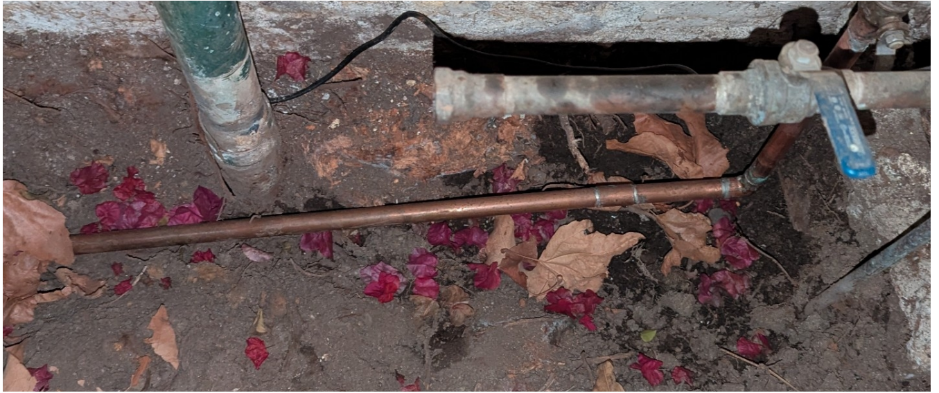
Picture 2: new pipe
