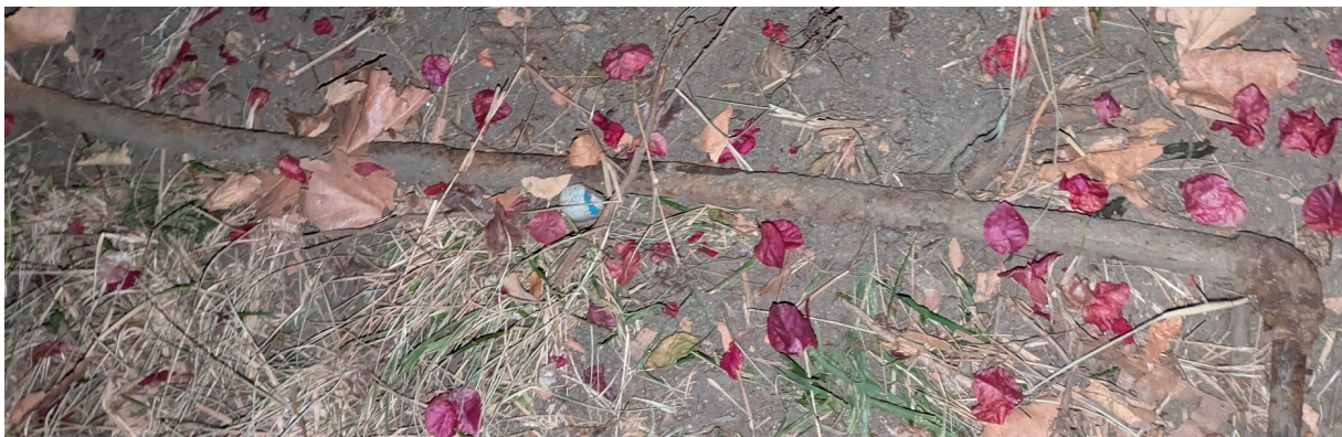
Picture 1: rusted pipe that leaked.
