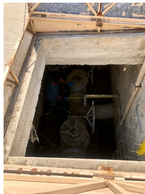
Figure 1 - Oak Creek 16-inch manifold. No flange or coupling on south end of the manifold
