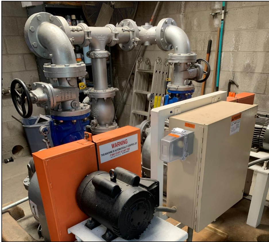
Figure 5-11: Lift Station Discharge Header
